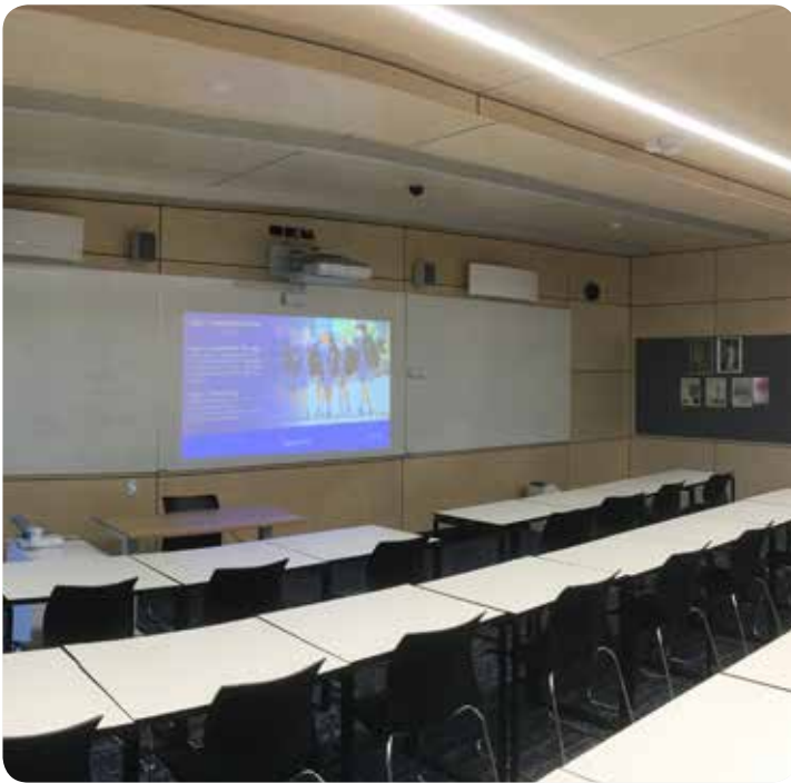
Epson EB-710Ui Full HD Laser Short Throw Interactive projectors were installed in the new PODS, along with Epson's ELP-DC21 Visualiser document camera, and VIVI wireless presentation solution for collaboration.
