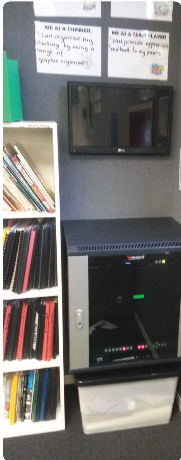
DiscoveryLab Preview Monitor and Equipment Rack
