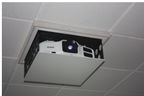
CCCC – Projector which recesses back into ceiling for flush finish
