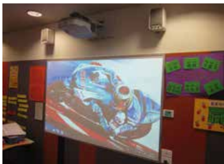
Epson interactive projector with JED control panel and tidy wall plate connections
