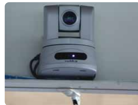
The HD camera used to capture the mass in the chapel
