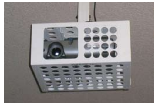
St Hilda's new wall-mounted projector housed in a protective security cage
