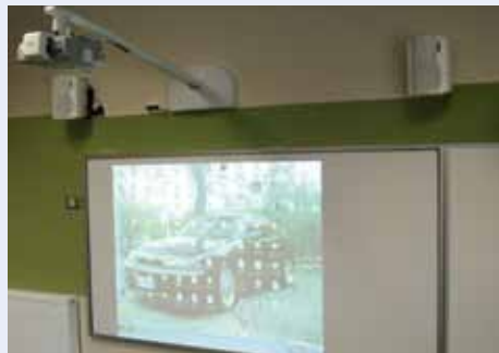
ABOVE: Having cabling roughed-in at the building stage results in a superior, more professional and aesthetically pleasing installation
