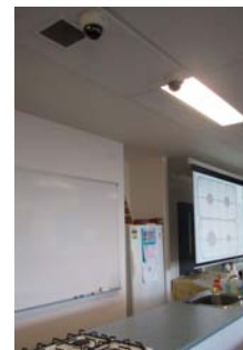
Above: Two high quality EVO 2 dome cameras installed over the demonstration bench
