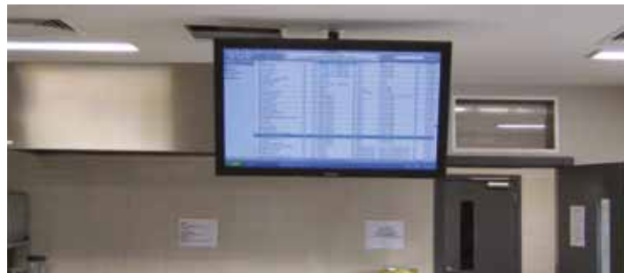
TOP: A Panasonic 50" HD (1024 X 768 Resolution) Professional plasma panel is installed in VET/Hospitality Kitchen at Penola Catholic College
